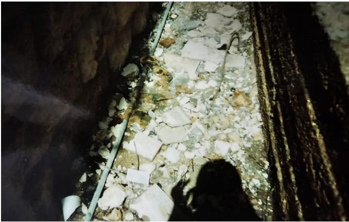
Rubble and shattered glass litter the floor beneath the damaged window, mixed with splintered plaster and fragments of the curtain rod. (Photograph by Mohammed Hijazi, Hebron, 2002.)
